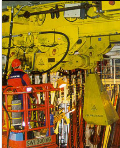
Location: SEA DRILLS Rig West Venture in the North Sea Application: BOP Handling System consisting of two JDN Monorail Air Hoists EHZ 75. Sender: Frode Ulriksen, Norway
